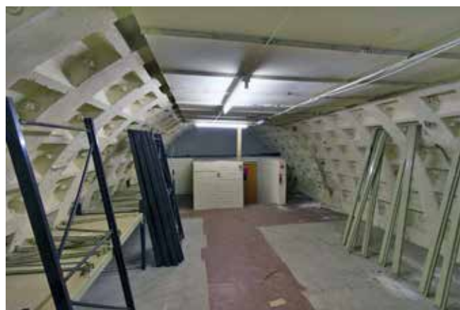
The north end of the upper level. From here stairs lead down to a cross passage to the parallel tunnel or to further stairs to the lower level
